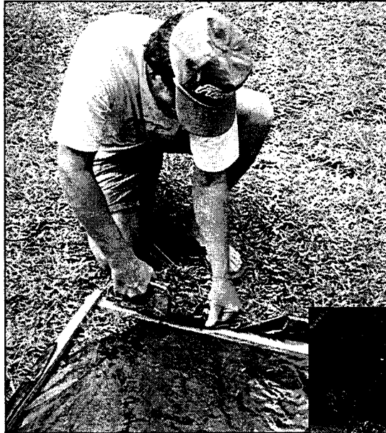
Above: Using a heavy duty stapler, the plastic sheeting was stapled to the frame. Notice the corners are left uncovered, so that anchors could be attached prior to being put in the water.
